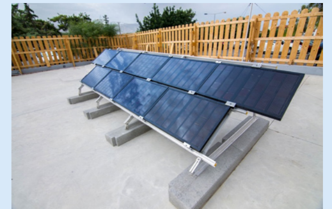
Solar farm installation at HMU, Greece, allowing the benchmarking of graphene-perovskite panels for commercial technologies. Credit: HMU/Emmanuel Kymakis
